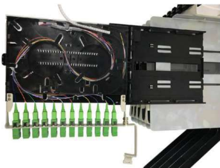
Double Sided Module System Storage Side
